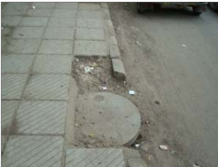
Magnum mismatch between round manholes and square tiles that plagues our city
