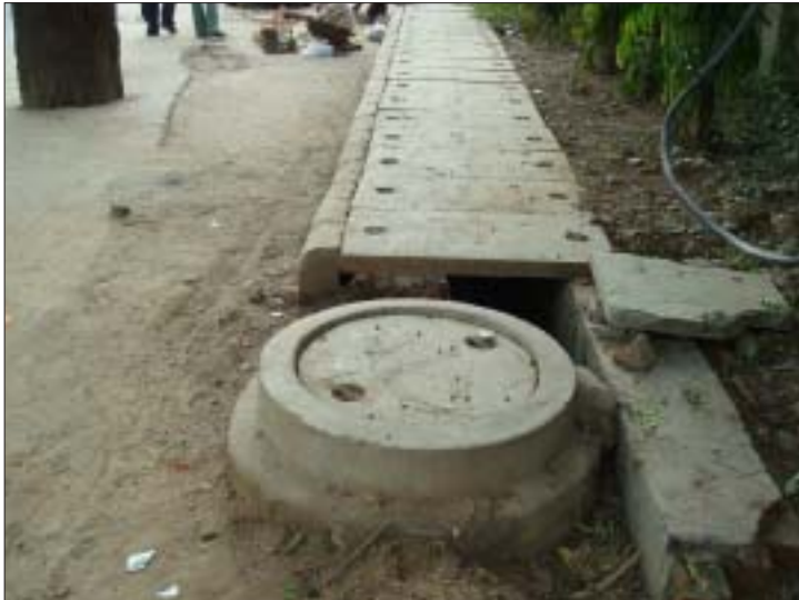
Absence of decisive methods to incorporate manhole into pavement stumps pavement makers and pedestrians alike
