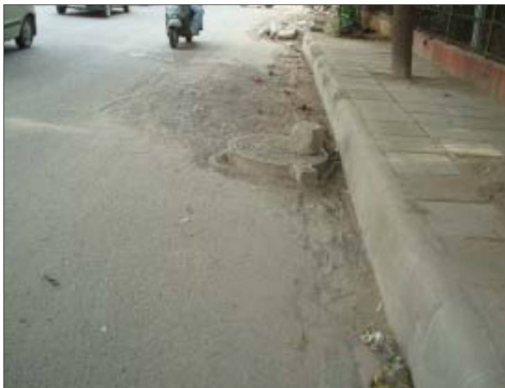
Raised manhole on road - a traffic hazard
