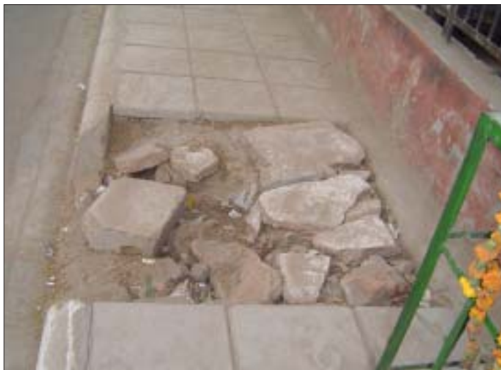
Storm drain left unpaved collects rubble in the middle of an otherwise perfectly paved pavement
