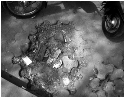
Fig. 5: The pavement tiles peeling off as the uncompressed ground beneath them begins to sink with time; photo taken by a student of St. Mary's School, New Delhi.
