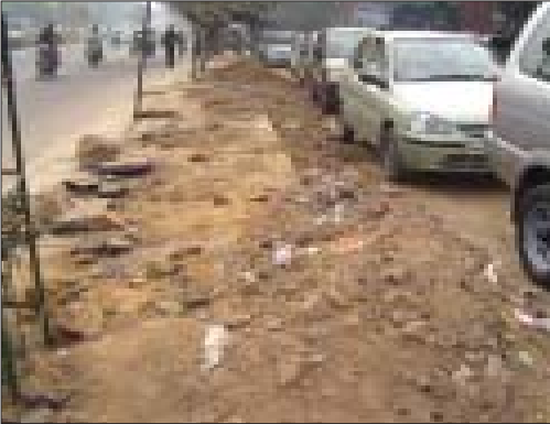
Undoing of a well done job: Dumping malba over a newly made pavement
