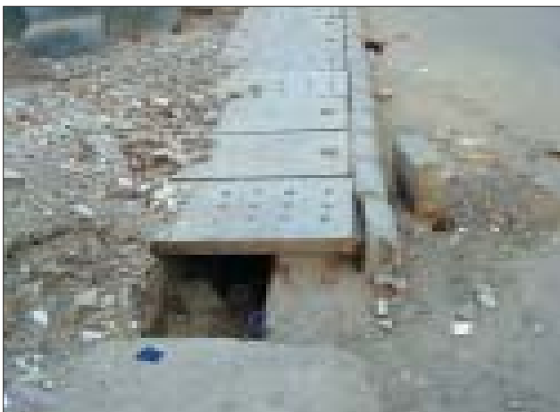
Malba spilling over brand new drain covers
