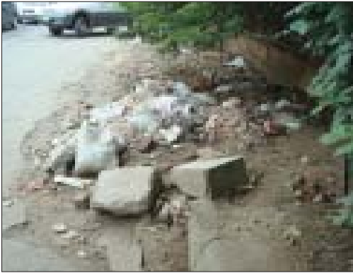
Good material gone bad: A disintegrated pavement
